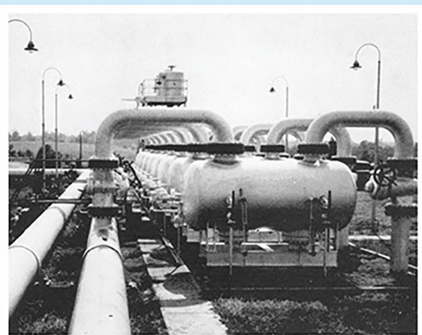
Battery of KingTool Gas Separator-Scrubbers with connections located to fit existing headers and valves.
